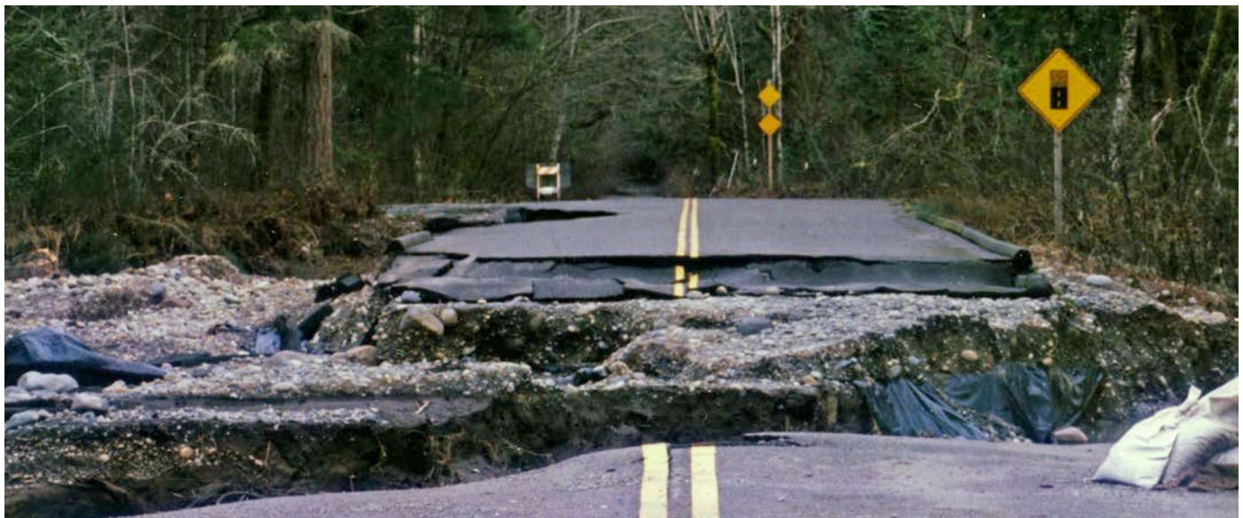
Kalama Creek access road flood damage, 2020
