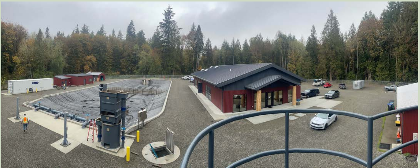
The Kalama Creek Hatchery is being totally rebuilt and modernized to meet the needs of current salmon enhancement.
