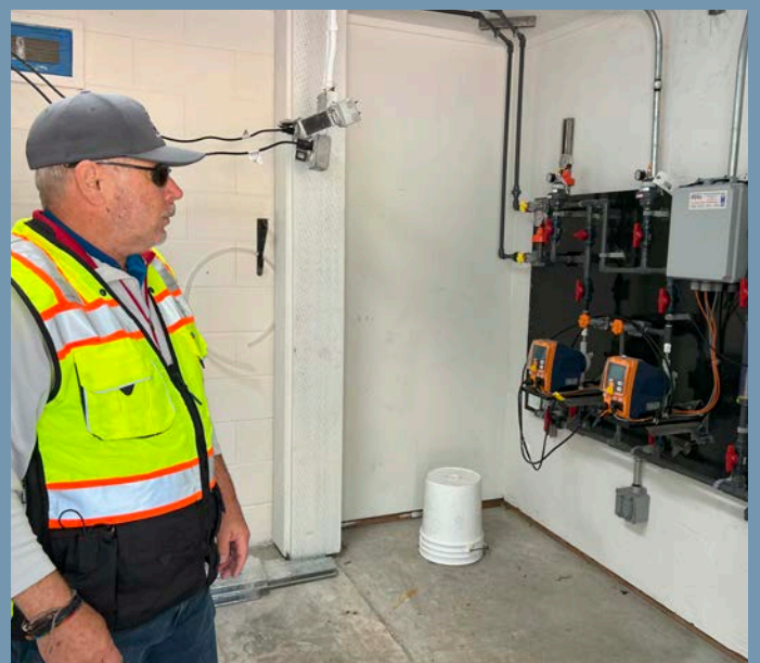
Public Works Director Tony Berkson inspecting new monitoring equipment installed as part of upgrades for Reservation water systems.
